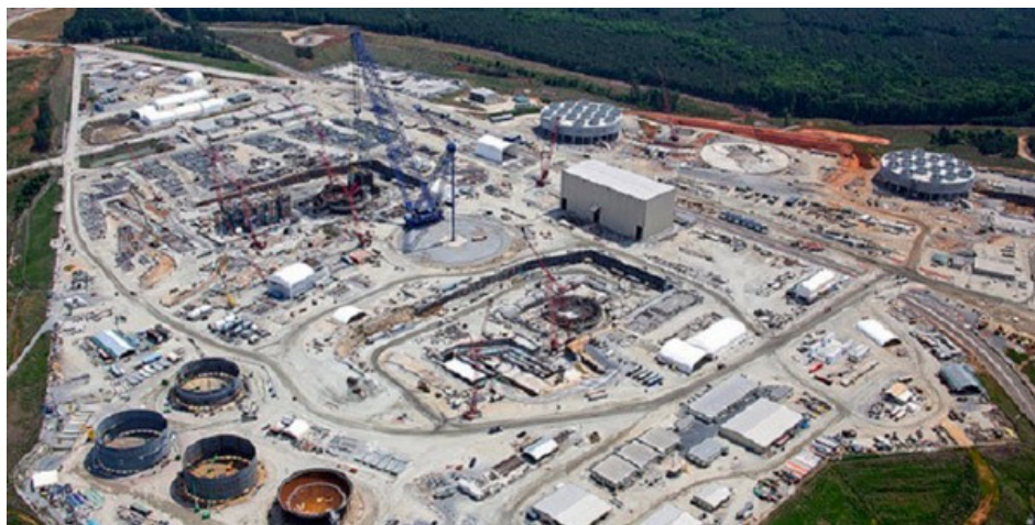
V.C. Summer plant construction in South Carolina. It's unclear if the plant will be finished after last week's bankruptcy filing by developer Westinghouse. | SG&E
